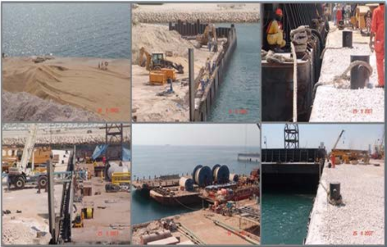
Project: Qcon Marine Yard Jetty Refurbishment Projects Client: Qatar Engineering and Construction Co. WLL Location: Mesaieed Industrial Area
